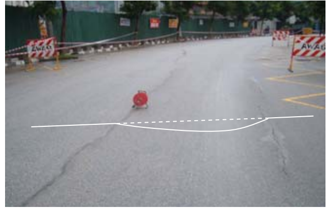
Fig. 10 Subsidence trough developed on the retained ground.
